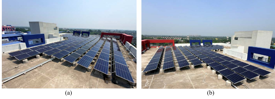
Figure 1. Practical rooftop PV system of total 182 panels on the (a) east side and (b) west side of the roof.
