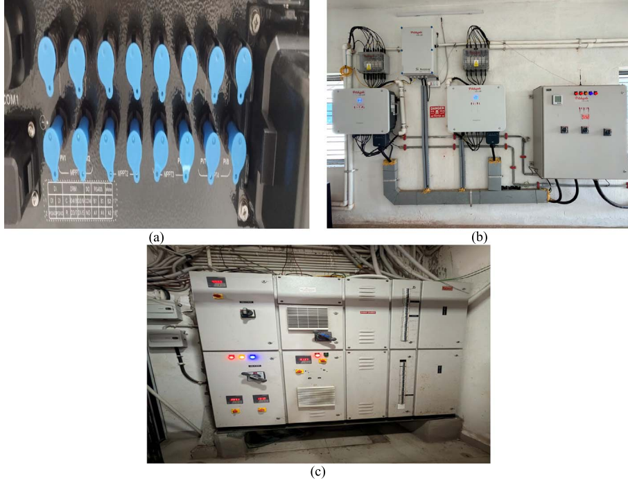
Figure 2. (a) MPPT provisions embedded in inverter casing, (b) DCDB, inverter and ACDB, (c) common bus bar where DG, PV and conventional supply are connected.
