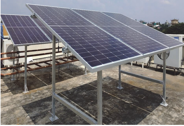
Fig. 3. Rooftop-mounted monocrystalline solar PV system.
